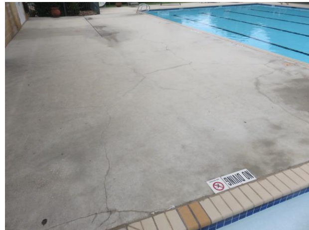
Unrepaired cracks throughout section of pool deck
