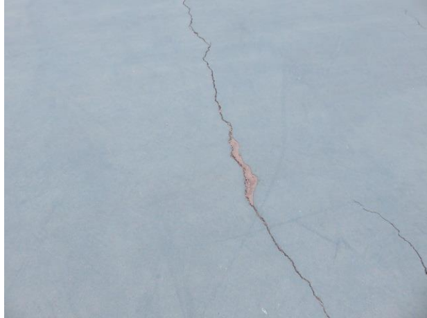
Wide cracks at tennis court
