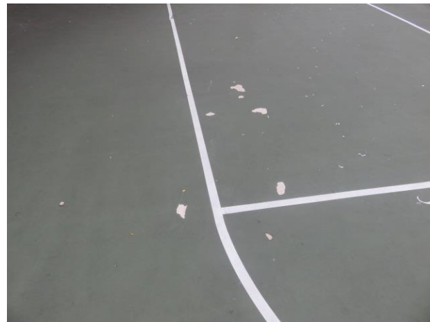
Color coat deterioration throughout basketball court
