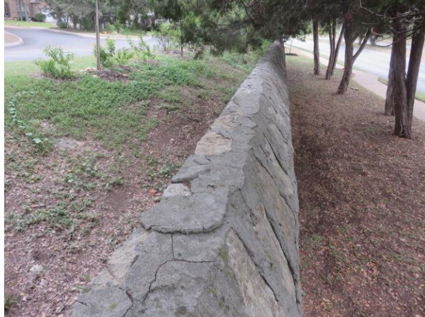
Topside of masonry perimeter wall with minor mortar deterioration
