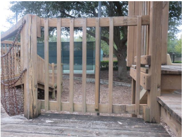
Missing spindle at playset railing
