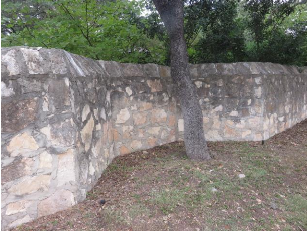
Front side of masonry perimeter wall (note proximity to tree roots)
