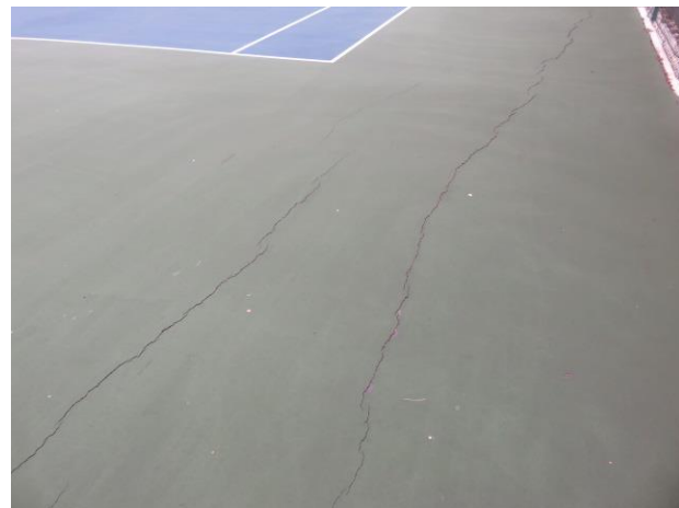
Typical cracks at tennis court edge
