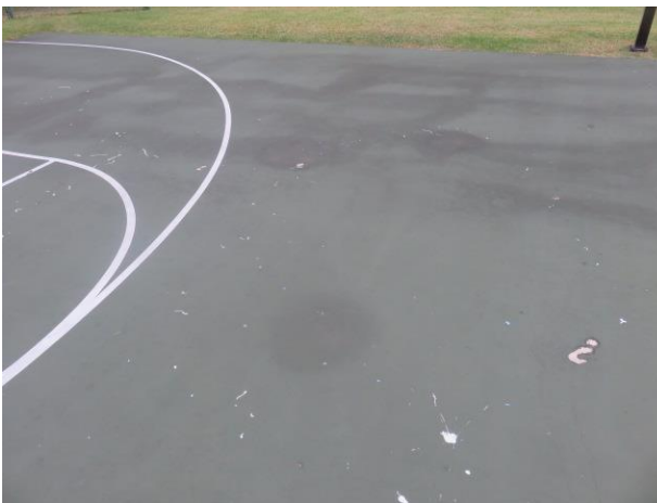
Color coat deterioration and evidence of ponded water
